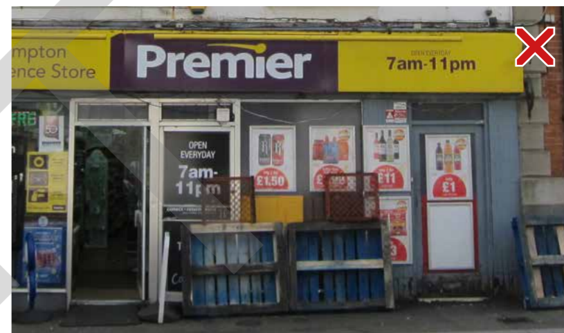
The shop front offers nothing to the street scene. No visual connection, no opportunity for lighting after hours, encouraging debris to be left against facade.
