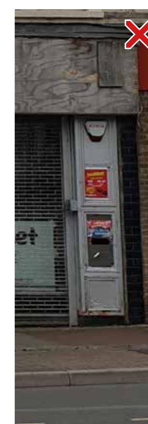
Original capitol overridden with enlarged fascia.
