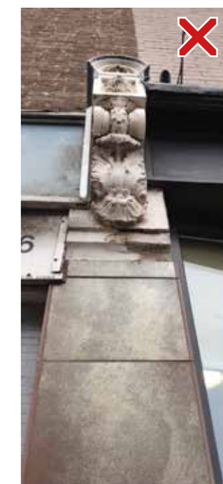
ornate corbel and capitol retained, inappropriate facing material placed on pilaster, with unsatisfactory detailing between old and new
