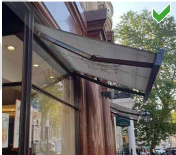
20th century metal shop front. Blind box incorporated at head of windows
