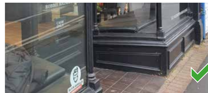
Original panelled risers stand proud of the window frame, with a protecting cill, sitting against internal structure which supports the glazing above.
